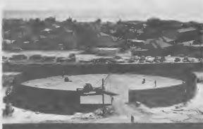
THE WALLS start up. From here, building tanks is like putting together a puzzle; every piece of steel has its place. E MURAYANAN ta cumenza bai larja. For di aki, trahamento di tanki ta manera trahamento di un rompecabeza.
